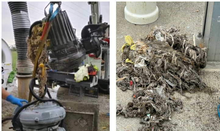
“Flushable” wipes clogging and damaging a sewer pump at one of Berea’s pump stations, resulting in repair costs >$50,000.
