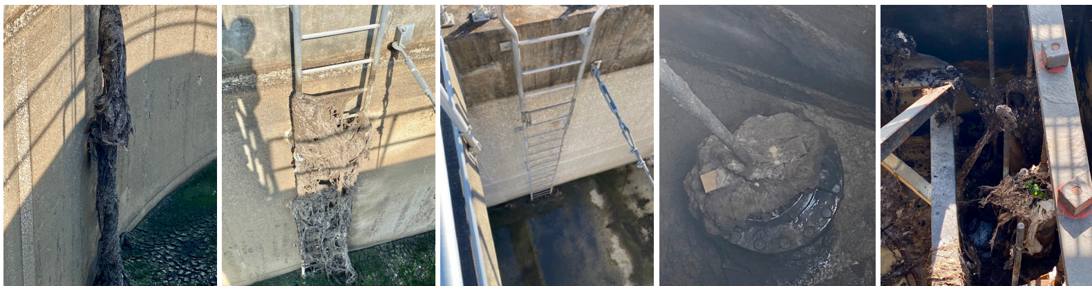
Problems resulting from “flushable” wipes at Berea’s wastewater plant, including covered valve stems, blocked access ladders, and clogged discharge pipes.
